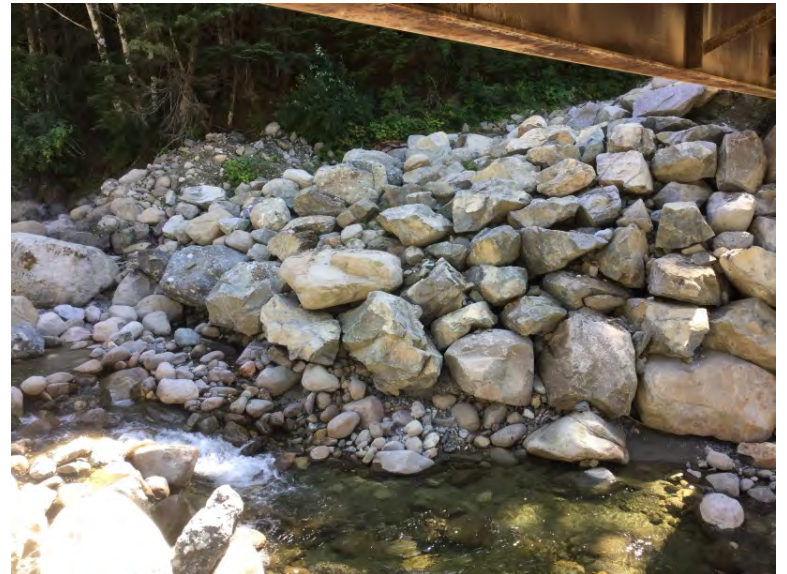
Upstream Left bank rip rap scour
