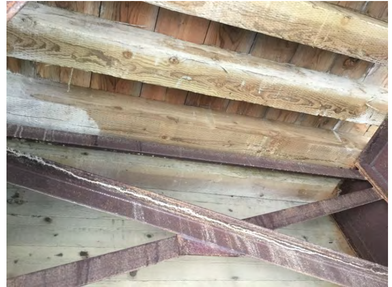
2nd tie right bank has minor check girder to girder
