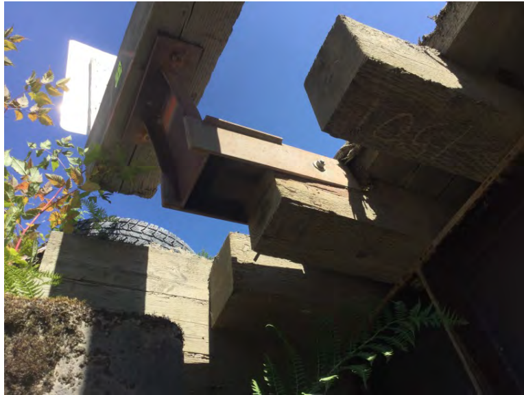
Downstream right approach rail damage
